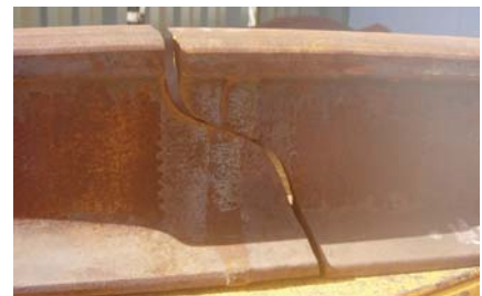
Close up of a rail which failed in the region of a weld
